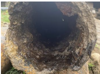
Water Main Pipe
