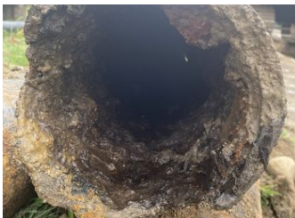
Water Main Pipe
